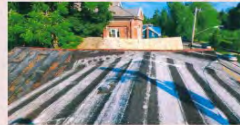
Above: 1 Albany Avenue roof current condition (Photo: William J. Better)
